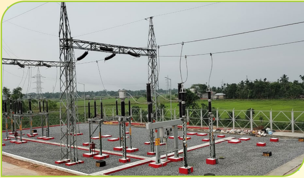
25KV Teliamura TSS, RE PKG-2 Silchar Project
