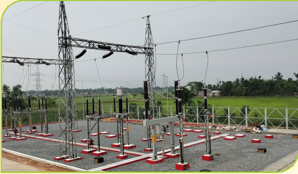
25KV Teliamura TSS, RE PKG-2 Silchar Project
