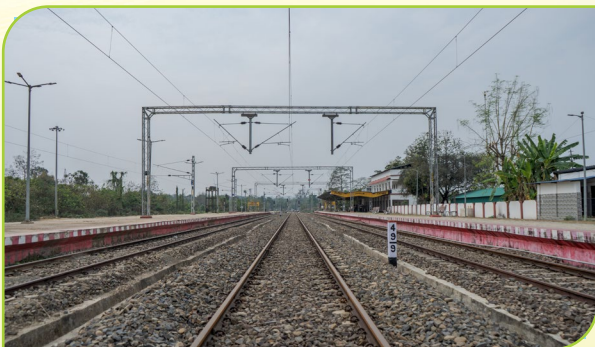
Jiribam Yard, Railway Electrification Pkg – 2
